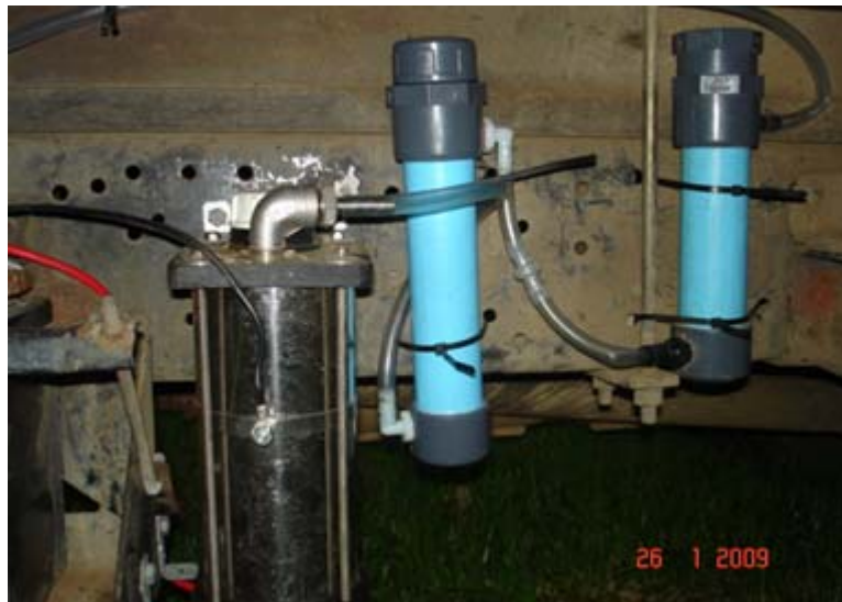
Booster installed with a water trap and safety bubbler
