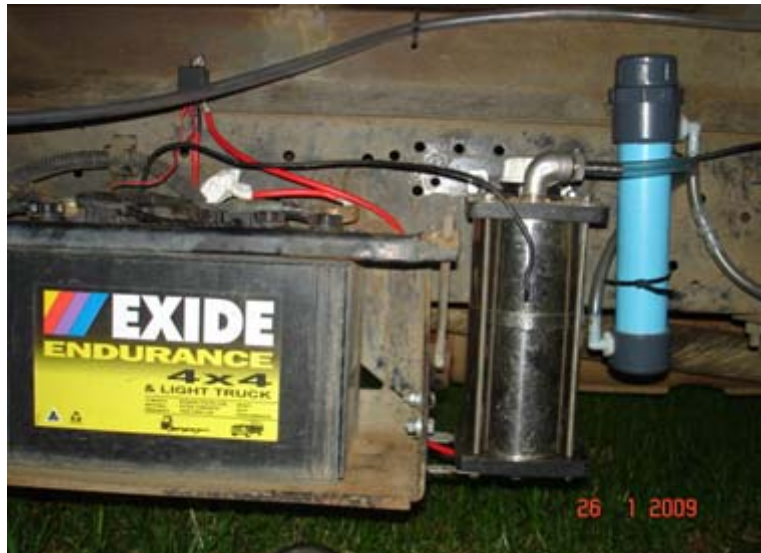
Relay installed on the left
